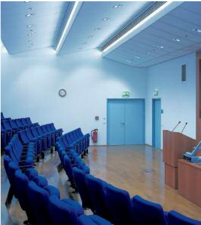
DALI controlled auditorium with Tridonic.Atco PCA Excel one4all ballasts
